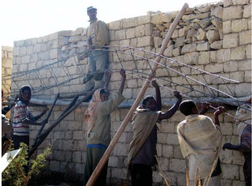
Community members at Dinwale village, Tigray, unite to place reinforcement bar in the frame of a Level 3 classroom.
